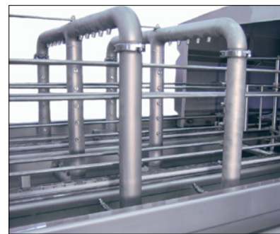
Tunnel Washer spray manifolds
